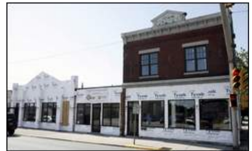
A new facade is in the works for the Monroe Circle Community Center at Western Avenue and Taylor Street, South Bend, where Granger Community Church is renovating these old storefronts.
